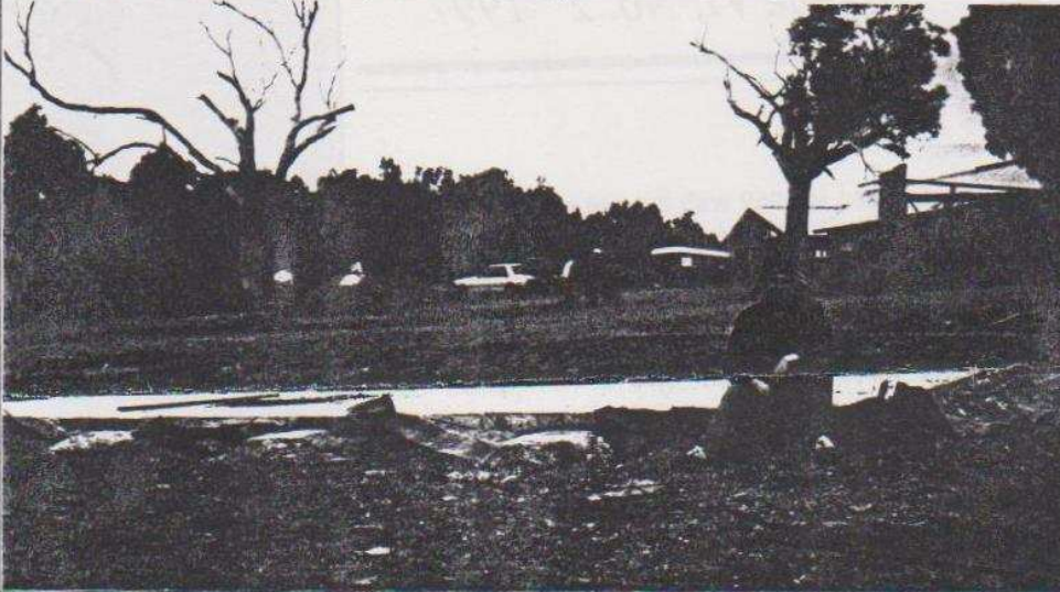
The roll-off roof Observatory concrete slab poured just prior to the first Working Bee at The Briars . The President poses while the grass is mowed and the earth moves.
